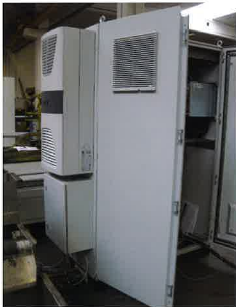
Air-condition in power supply box
