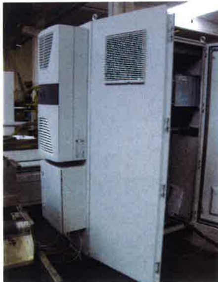
Air-condition in power supply box
